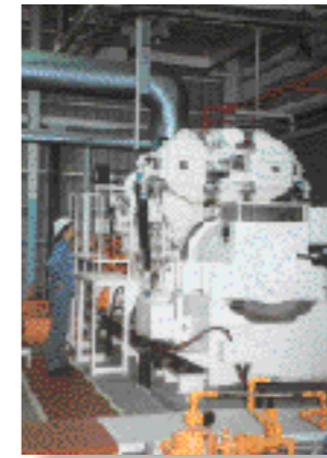
Effective utilization of thermal exhaust
